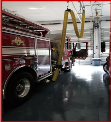
X-6: Fire apparatus connected to a source capture vehicle exhaust extraction system.
